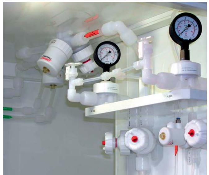
Detail of a chemical supply system
