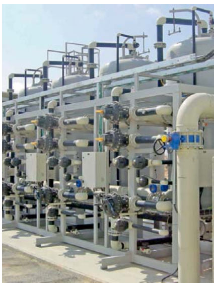
Water treatment (company Treitel Chemical Engineering LTD)
